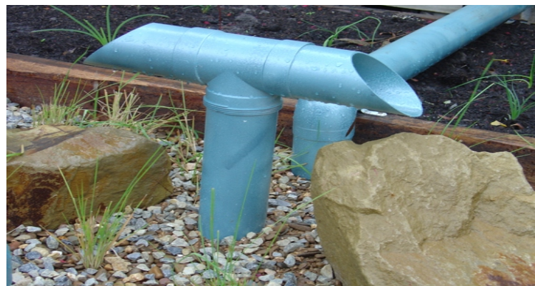
This is a photograph of the Raingarden at Armadale Primary School designed by Ruth Czermak (Botanical Traditions). A Raingarden is a special area which is constructed to filter rainwater and remove nitrogen, phosphorus and suspended solids. It also helps to reduce the velocity and volume of water entering our creeks and rivers in storm events.
